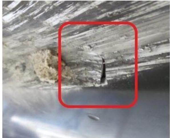
Figure 3 – Visible open crack
