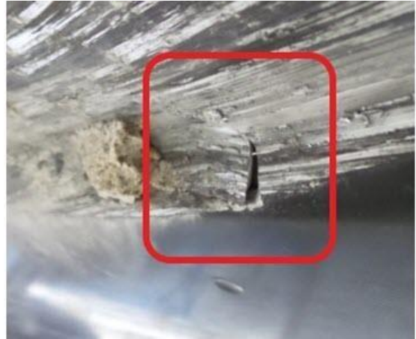
Figure 2 – Visible open crack
