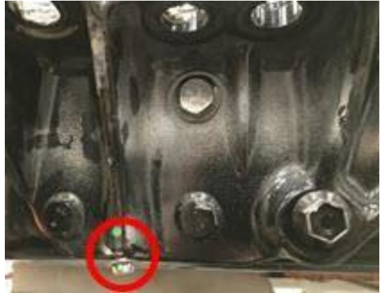
Figure 12 – Skid plate to doubler fastener sheared/bent
