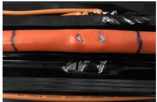
Figure 17 – Damaged cable under center ski
