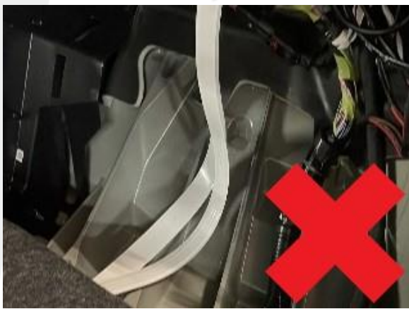
Figure 18 – Incorrectly routed through RH channel
