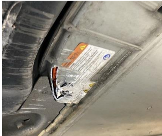
Figure 1 – Rupture of the enclosure exposing internal electronics
