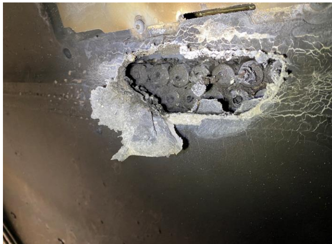
Figure 21 – Heat exposure causing enclosure rupture with internal components exposed
