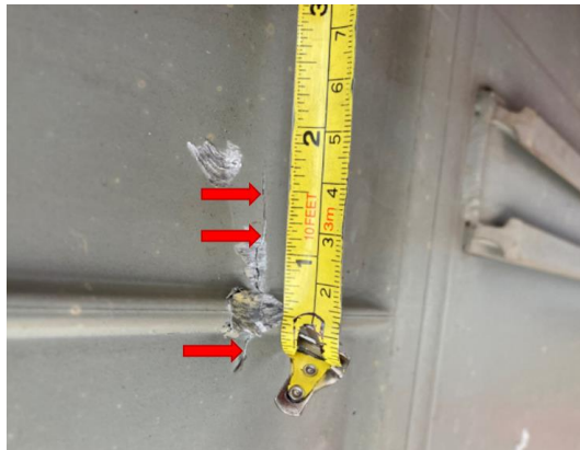
Figure 4 – Large enclosure crack breaking the enclosure sealing
