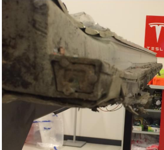
Figure 15 – Enclosure visually bent
