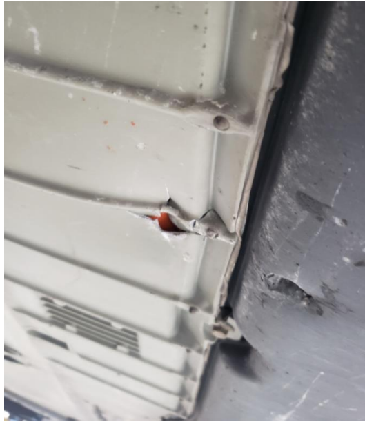
Figure 3 – Enclosure underside rupture exposing internal components
